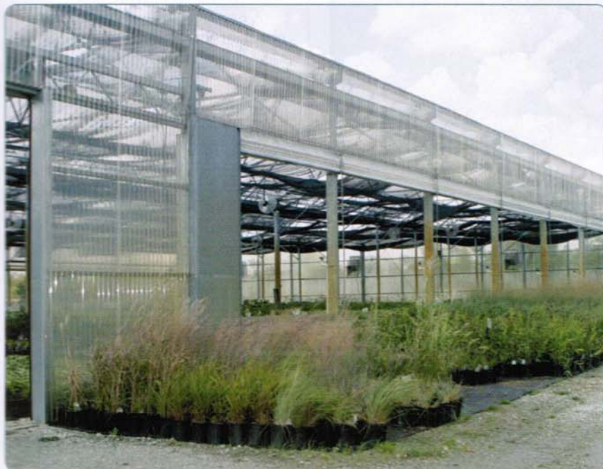
Perennials Plus expanded its growing space to some outdoor pads after one of its greenhouses collapsed.
